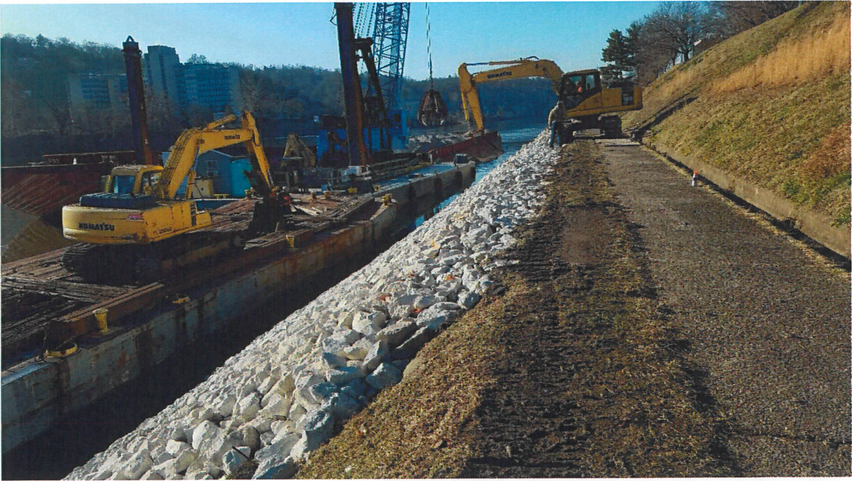
Figure 1 Representative slope protection work being performed during initial phase of the LRH Kanawha River, Greenbrier Street CAP 14 project. Photo location: Charleston, WV directly upstream of the current Elk Option.
