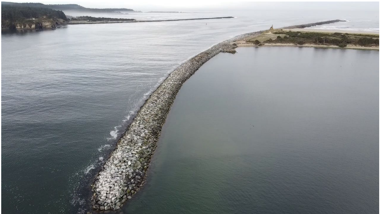
Aerial photograph of the Coos Bay North Jetty tail from above in August 2025. Courtesy of USACE.
