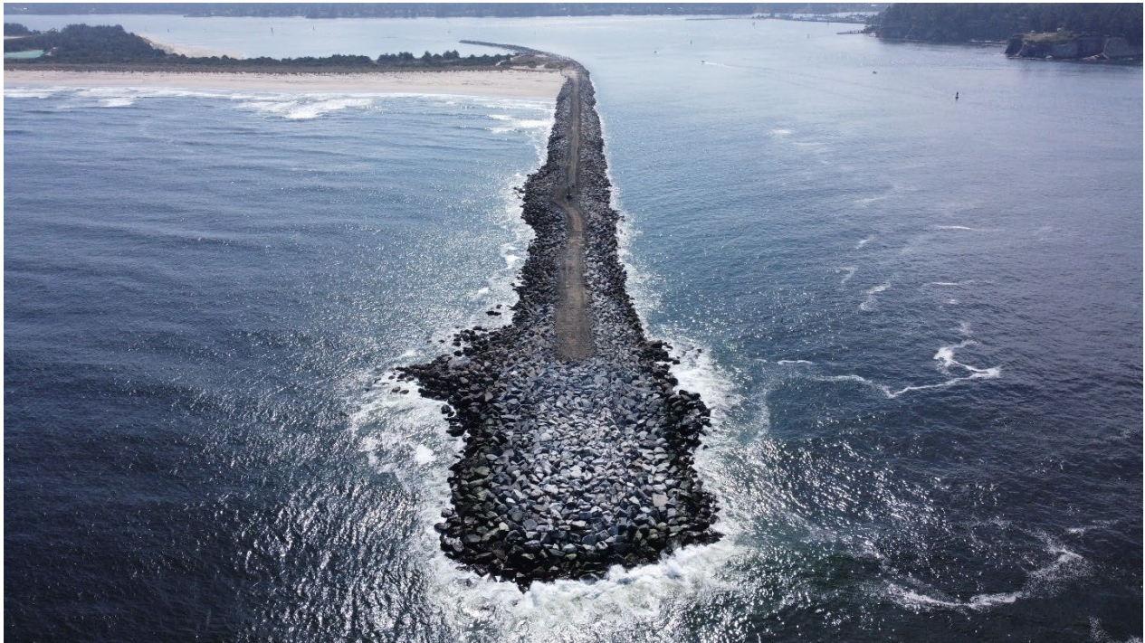
Aerial photograph of Coos Bay North Jetty head in August 2025. Courtesy of USACE.
