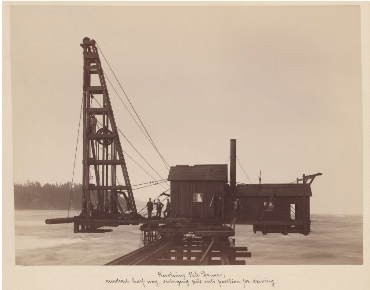
Pile driver used during construction of Coos Bay North Jetty tramway. Photograph by J.H. Bratt, 1892. Courtesy of Library of Congress.
