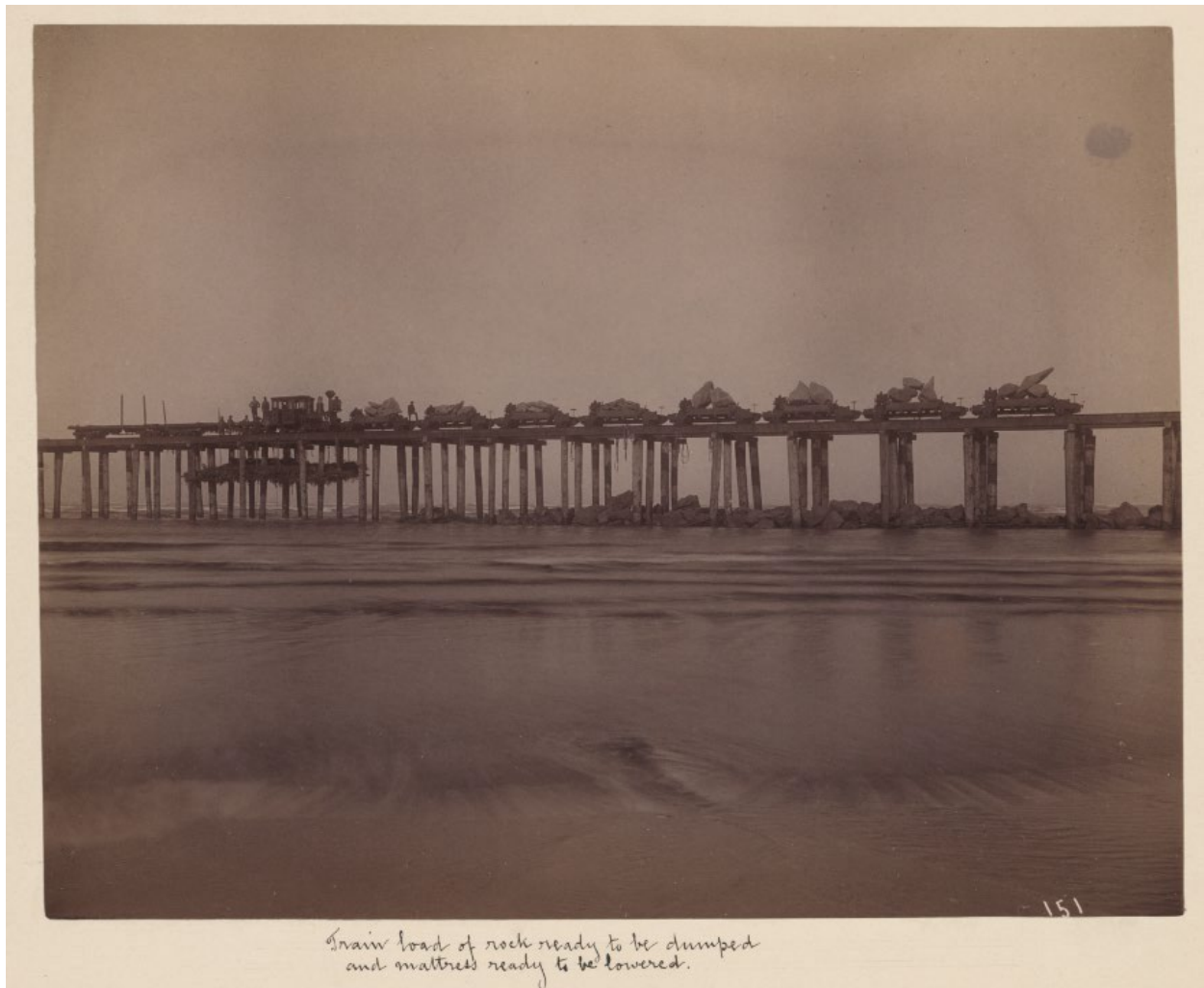
Coos Bay North Jetty elevated tramway loaded with rocks and brush mattress during construction. Photograph by J.H. Bratt, 1892. Courtesy of Library of Congress.
