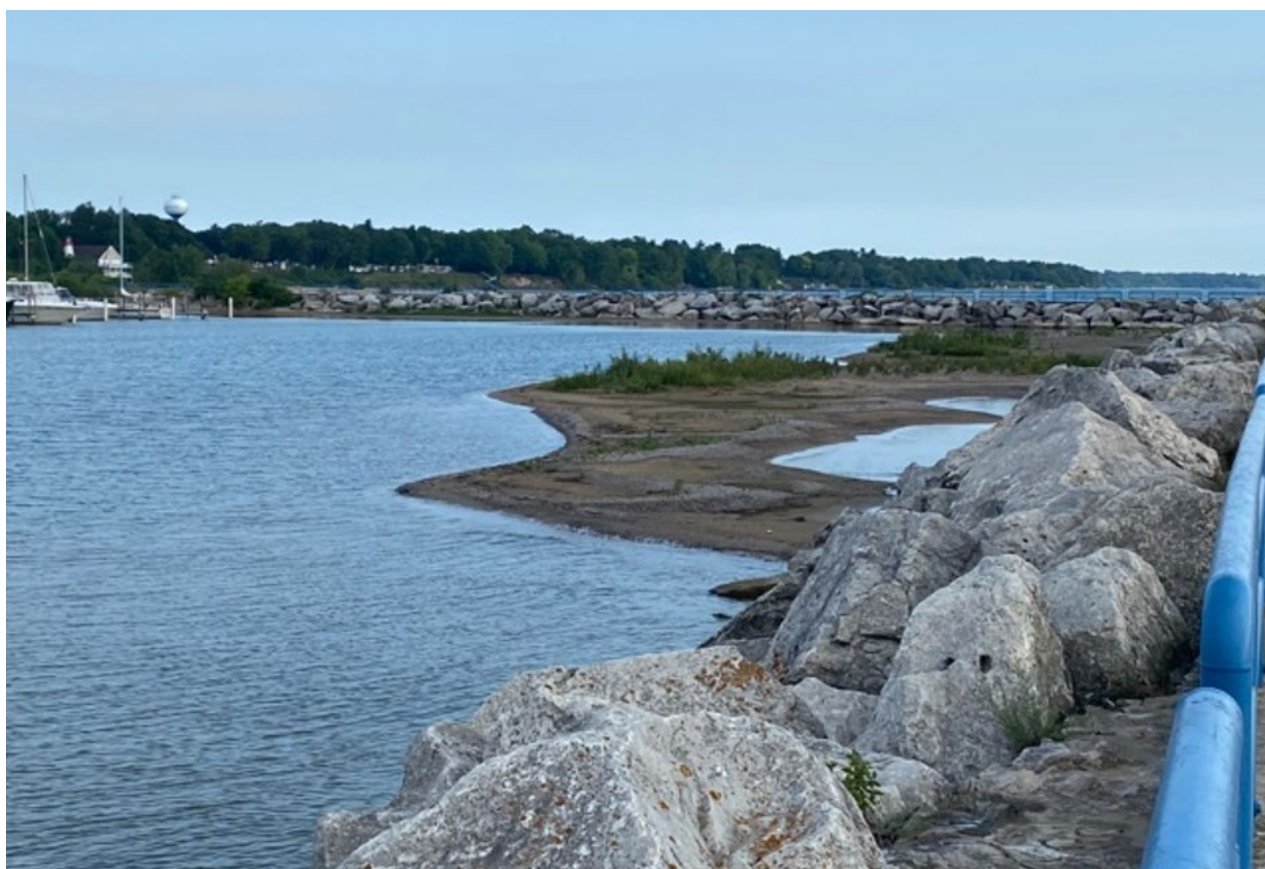
FIGURE 3. SEDIMENT INFILTRATION THROUGH LEXINGTON NORTH BREAKWATER
